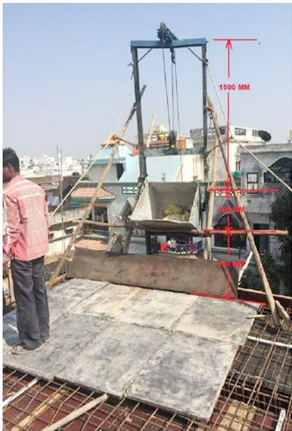
Fig. 3: Fig. of real time elevator with vertical distance.
