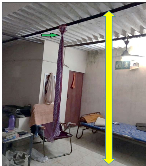
Figure 2: Scene of the incident showing the ligature material (Green arrow) tied to the ceiling beam with a chair placed beneath it (Yellow arrow showing the height of the ceiling beam from the floor- 8.5 feet)
